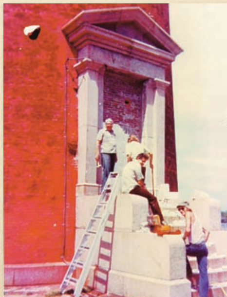
THE SEALED FRONT DOOR OF THE TOWER IS OPENED AS REPAIRS BEGIN
