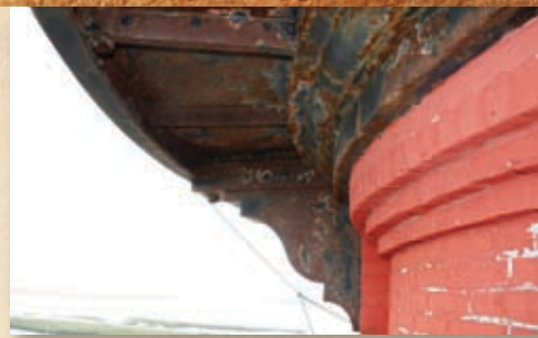
THE GALLERY DECK BEFORE CORROSION IS REMOVED
