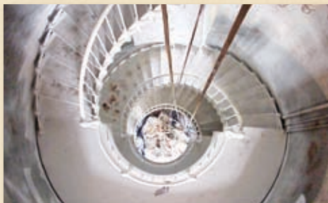
ALL IRON WORK WITHIN THE PONCE INLET LIGHTHOUSE WAS FULLY RESTORED IN 2001
