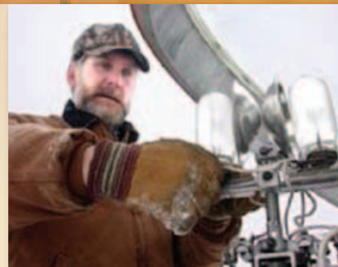
MIKE ROGAN INSTALLS A NEW LAMP IN THE BEACON AT MACDONALD PASS. COURTESY OF MIKE ROGAN
