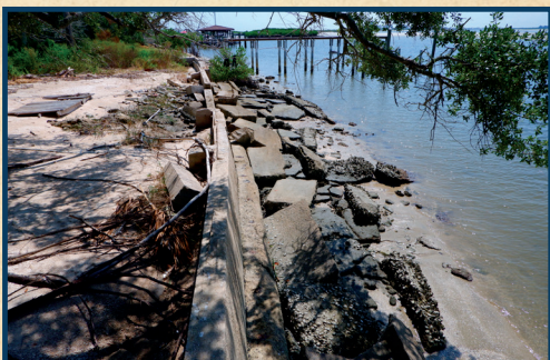
The damaged sea wall resulted in shoreline erosion
