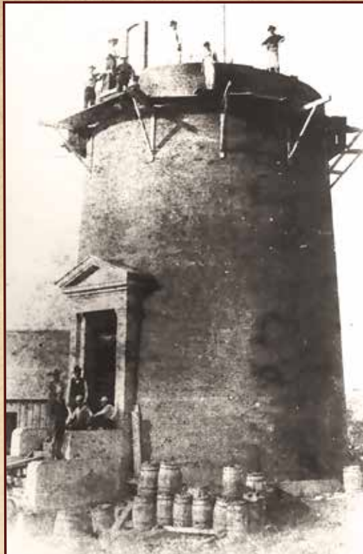
This photograph clearly shows Herbert Bamber's revolutionary "working platform" being used by masons during the construction of Mosquito (now Ponce) Inlet Lighthouse. Prior to its invention, most masonry towers were built using traditional scaffolding systems.
