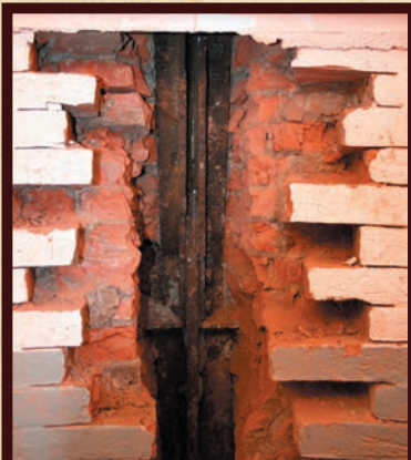
With the lantern room tie down rods exposed for the first time since 1887, Federal Masonry employees could address the corrosion issues that had caused hairline cracks to form in the watch room masonry walls.
