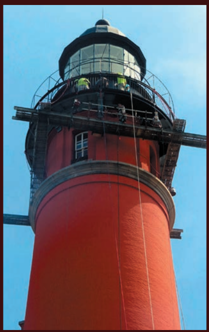
Accessing the top of the tower via a lift stage, Razorback LLC employees clean, treat, and repaint the underside of the gallery deck and its support brackets.
