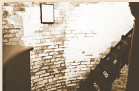
THE LIGHTHOUSE'S INTERIOR IN NEED OF RESTORATION
