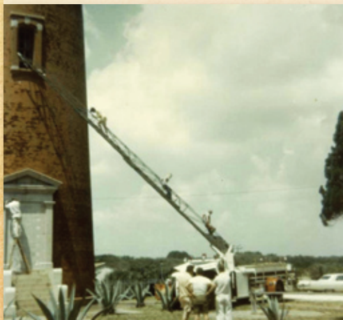
IN 1972, ACCESS INTO THE LIGHTHOUSE WAS ACHIEVED USING AN OLD FIRE TRUCK
