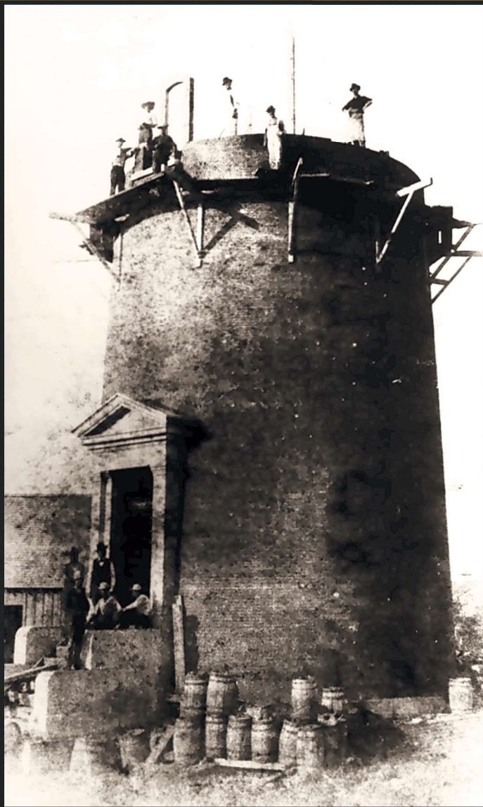
The Mosquito Inlet Lighthouse under construction, c. 1886; Note the casks of bricks at the base of the tower and the window frame being set in the wall. Image part of the Ponce de Leon Inlet Lighthouse Preservation Association collection.
