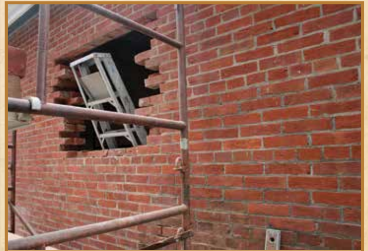
The hole is prepared for restoration using historic bricks from the original construction of the Light Station
