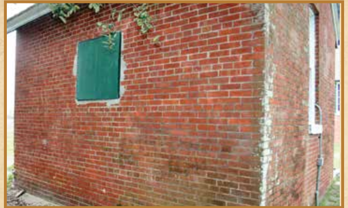
Many years ago a hole was cut in the east wall to accommodate an air conditioner.
