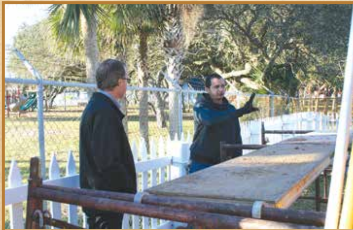
Ed Gunn, executive director of the Light Station, confers with Jonathan Leonor, leader of the Federal Masonry crew.
