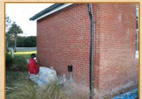
The west wall has been completed and work on the north wall is underway.
