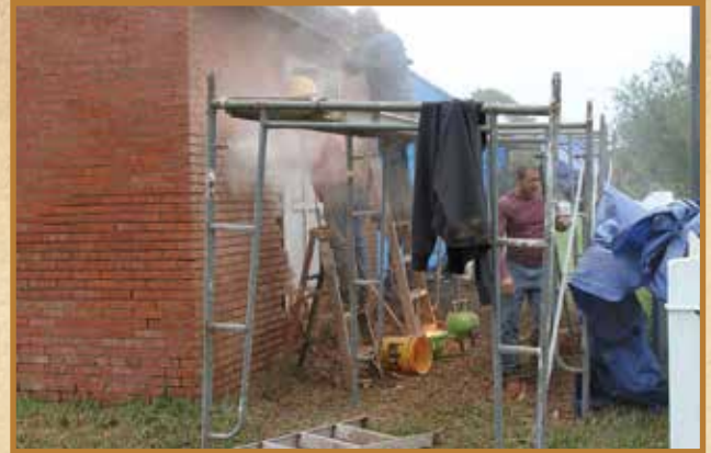
Jonathan Leonor dodges the dust as repair of the south wall begins.
