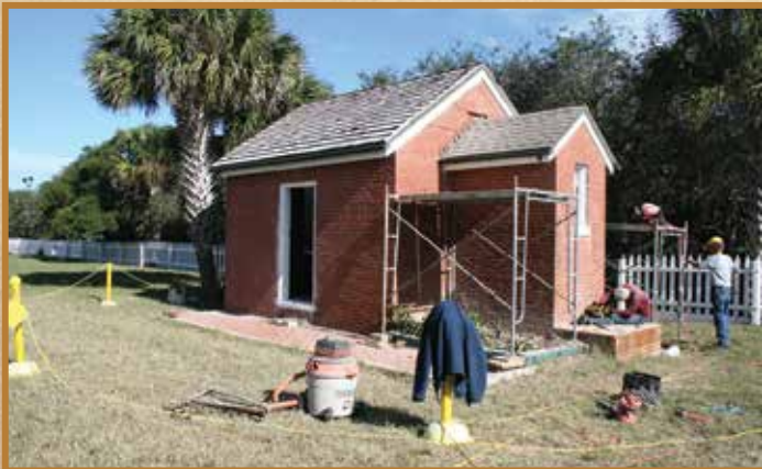
The crew begins the project with the principal keeper's woodshed and privy.
