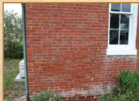
West wall of the Woodshed Theater before repair.
