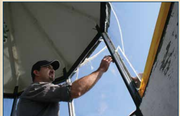
Mike Bennett measures a lantern room window as a possible exit point for the lens.
