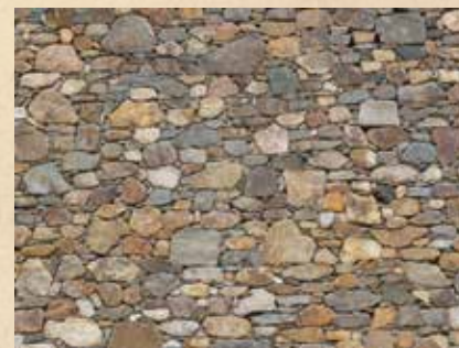
Most Colonial-era lighthouses were built of uncut stone shards or river rock commonly referred to as rubble stone.
