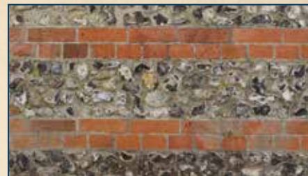
Rubble stone and fired brick was often used together in the construction of walls and buildings. This wall was built by the Romans more than two thousand years ago.
