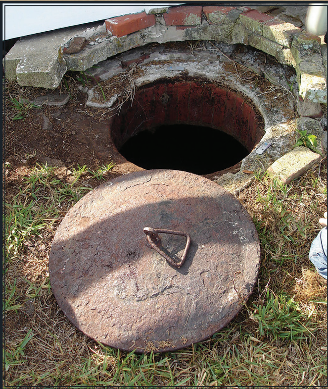
Access lid to the second assistant keeper dwelling cistern; collection of the Ponce De Leon Inlet Lighthouse Preservation Association.
