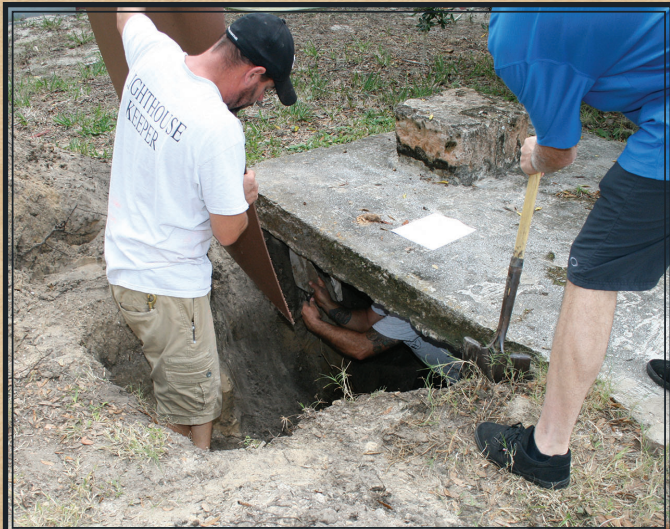
Ed Gunn (right), Tom DiTusa (in hole), & Michael Thorpe (left) begin restoration work on wall of cistern #1; collection of the Ponce De Leon Inlet Lighthouse Preservation Association.
