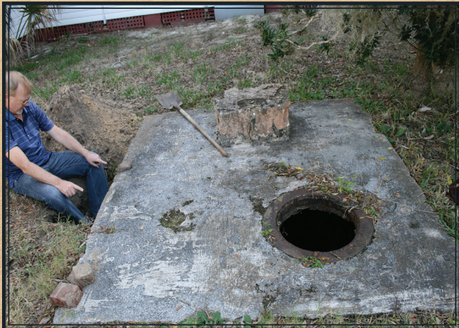
Executive Director Ed Gunn estimates size of the large hole in cistern #1 prior to making restoration repairs; collection of the Ponce De Leon Inlet Lighthouse Preservation Association.
