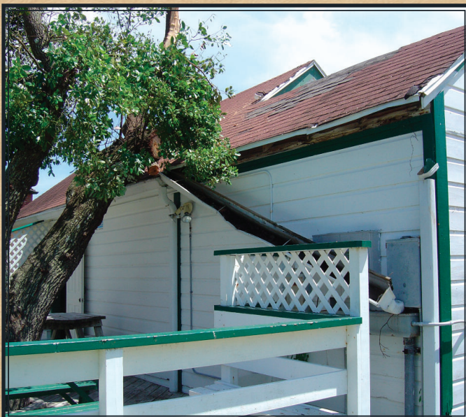
Gutter damage after Hurricane Charlie in 2004; collection of the Ponce De Leon Inlet Lighthouse Preservation Association.
