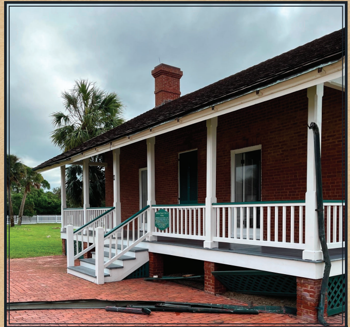
Damaged Gutters Caused by Hurricane Ian
