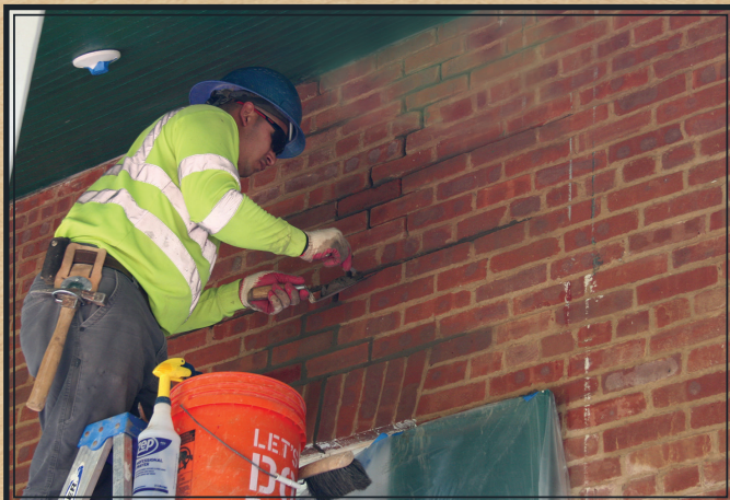
Lead mason Jonathan Leonor repoints the mortar joints above the 1st Assistant Keeper dwelling's small bedroom window.
