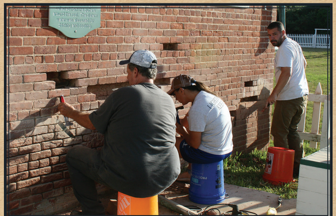
Chuck Spitznagel, Maintenance Manager Quincie Wend, and maintenance employee Mike Thorpe restore the 1st Assistant Keeper dwelling's south wall in May, 2022.
